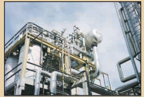
IsoTherming™ reactor in first commercial ultra low sulfur diesel unit, Gallup, NM.
